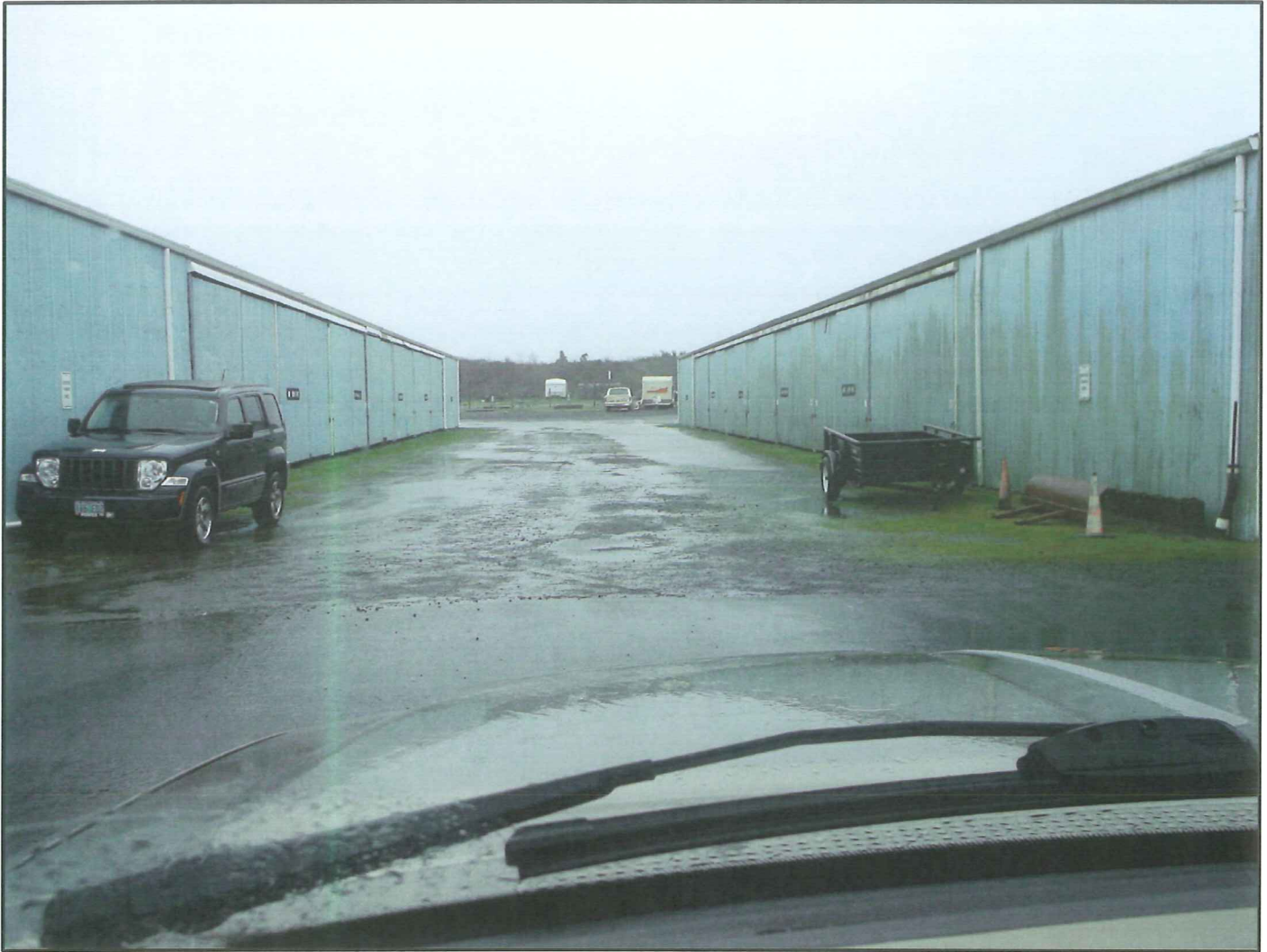
Standing water between the two storage buildings, looking east.
