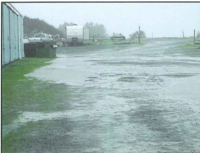
Standing water on south side of storage buildings.
