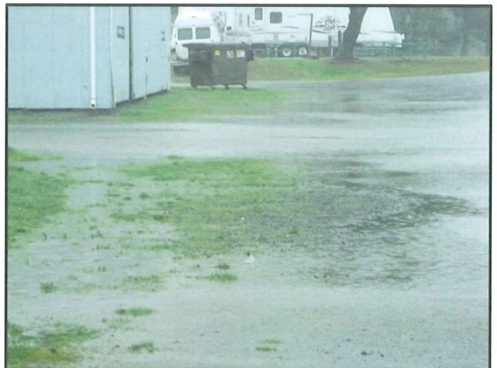
Standing water on east end of storage buildings.
